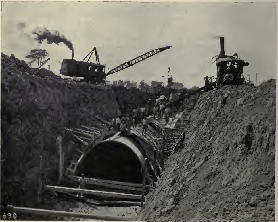
A BUCYRUS DRAG-LINE BACKFILLING ON THE WETHERBY SEWER, DETROIT, MICH. Blaw-Knox collapsible steel forms are being used on this job by the contractors, Nash Brothers, Chicago, Ill.
